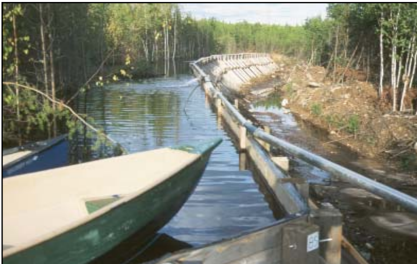
A portion of the wooden dike enclosing upland reservoir 3, with sampling boats floating on the reservoir surface. The water at this location is approximately two metres deep. The pipe running along the top of the dike carries water pumped from nearby Roddy Lake to keep the reservoir filled.
