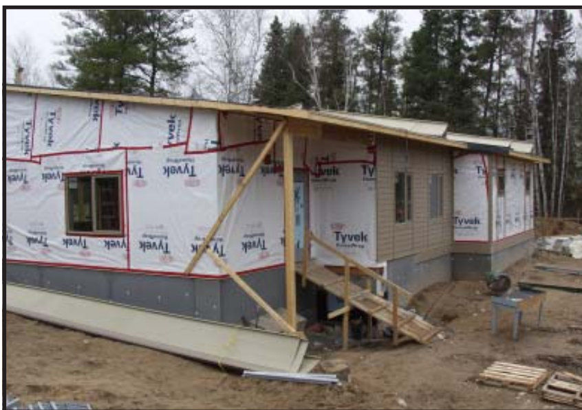
One of the two new dormitory buildings under construction in April 2006. These buildings are replacing several original trailers and frame buildings.
